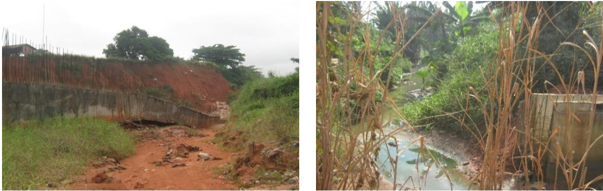
Plate 11: Failed Engineering Intervention at Queen Ede Gully erosion site/West Moat catchment in Benin City
