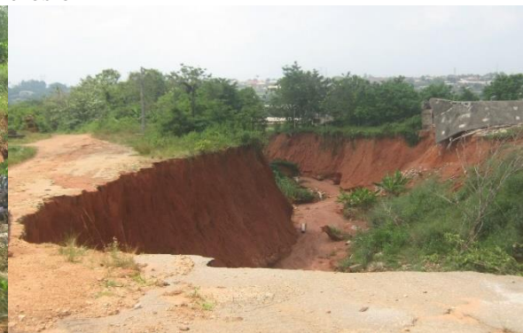
Plate 10: Erosion off major road in Ekehuan, Benin City
