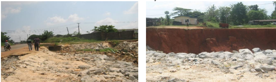
Plate 12: Failed Engineering Intervention at Ekehuan erosion site, in Benin City
