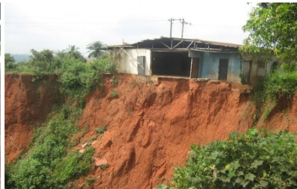
Plate 8: One of the residential buildings in Ogbeson quarters being threatened by Queen Ede erosion
